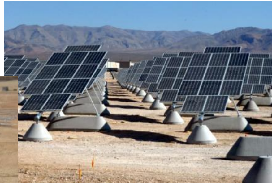
SunPower T20 Tracker at Nellis Airforce Base
