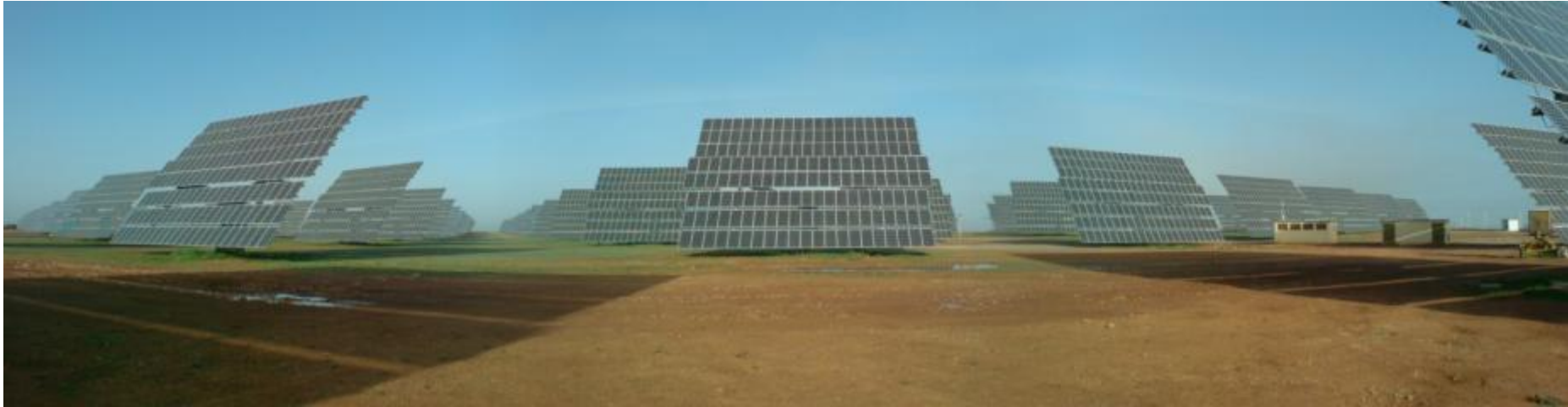
Arsol 1 (5MW) ARIES PV Plant
