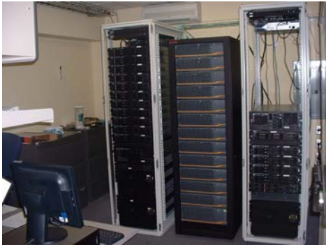
Server (19) and Storage (51 TB) racks
