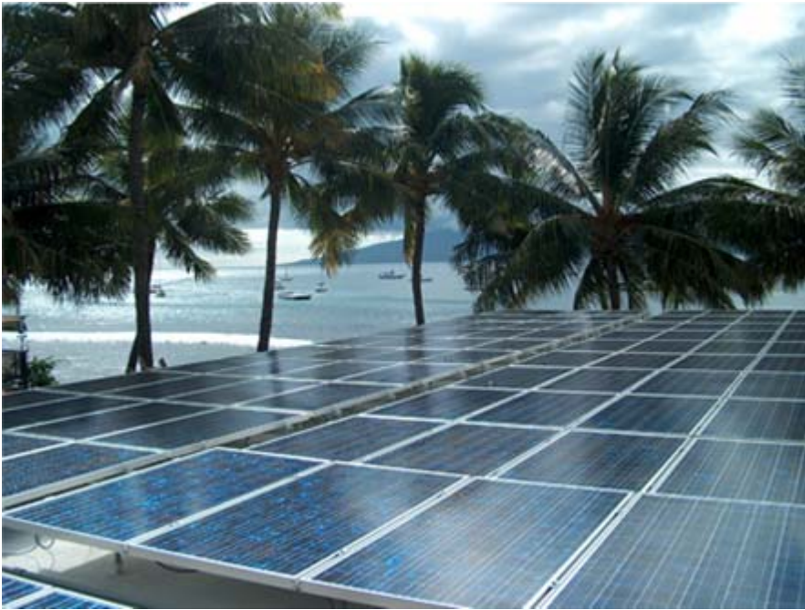
19.8-kWp Commercial system in Hawaii by ProVision Technologies
