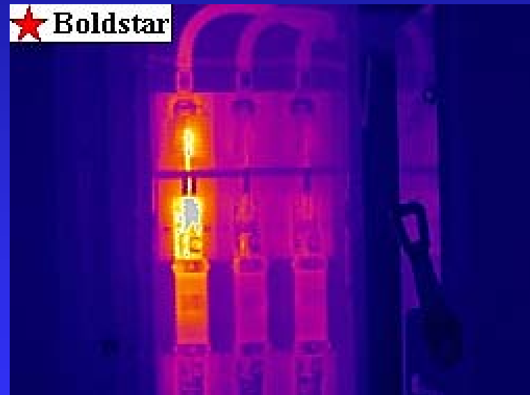
Overheated of disconnect switch
