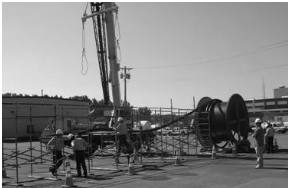
Fig.15. Installation of the 30 m long cable made by Sumitomo Electric with nearly 10,000 m of SuperPower's 2G HTS wire.
