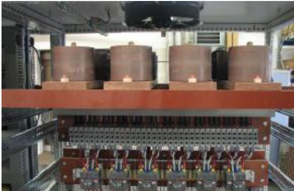
Fig. 6. Power distribution unit of the 5 kWh HTS FESS
