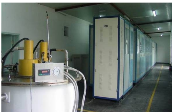
Fig. 19. The 1 MJ/0.5 MVA HTS SMES system.
